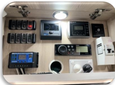
Main switch board panel located inside the cabinet.
